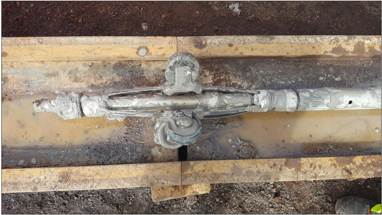
Figure 14. The lower centralizer of the CBL-probe after the CBL-log on July 31 st in well K-41.
