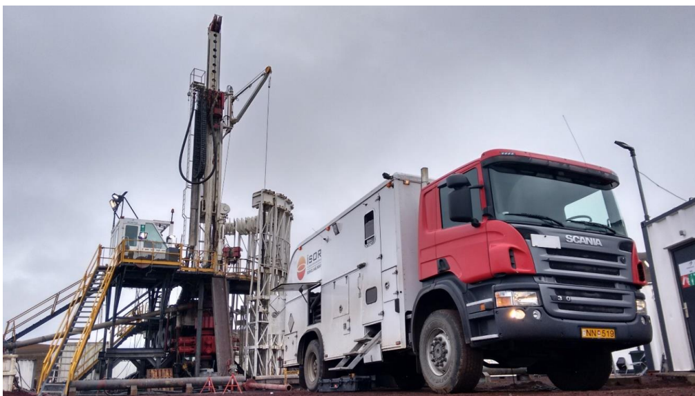
Figure 1. The logging engineers arrived early this morning to carry out a gyro-log inside the drill-string in K-41.
